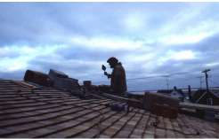
Contad Malicouat, level raised, ready to start work on the chimney as it comes through the roof at 86 Commercial Street - 1977
