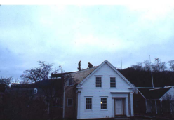
Conrad Malcool and helper as the 7 flue chimney is ready to come through the roof - 1877
