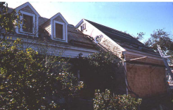
East side of 38 Commercial Street in 1977 as exterior work was in progress
