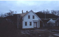
38 Commercial Street in 1977 undergoing renovation - Conrad Malicoal and his helper on the roof as they prepare to have the chimney come through
