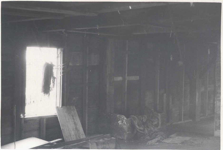
Atlantic Coast Fisheries Cold Storage Trap Shed on Freeman's Wharf -Interior before demolition, winter, 1974 (photos by Josephine Del Deo)
